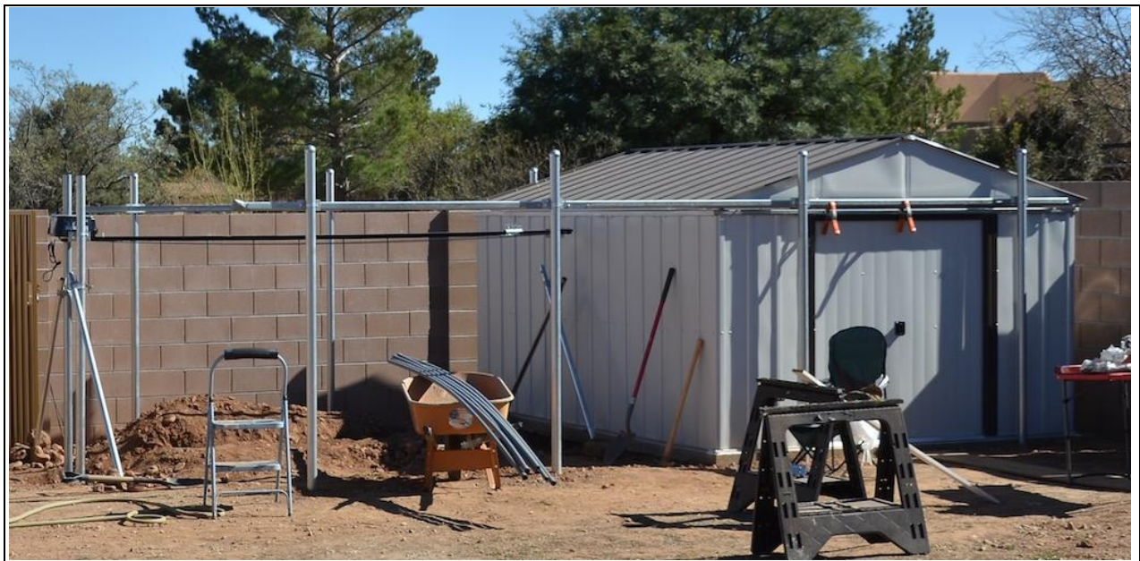
Figure 14- Modified Arrow Shed Roll-Off Observatory with Partially Complete Roof Tracks and Opener
