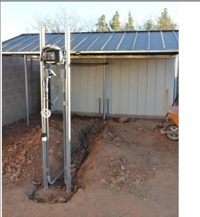
Figure 15- Supports and Conduit for Garage Door Opener
